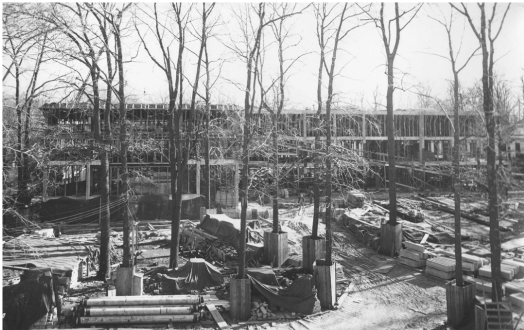
Figure 29. During the construction of Bowditch Hall, 1942 (USMMA Bland Library). Note protective fencing around mature trees to prevent damage during construction.
