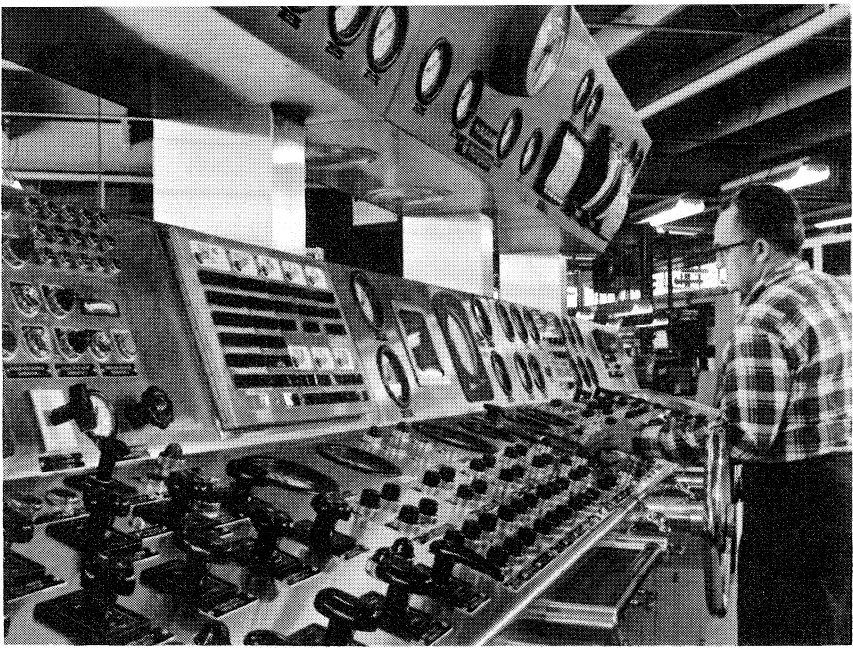
The control console of a mechanized engine room.
