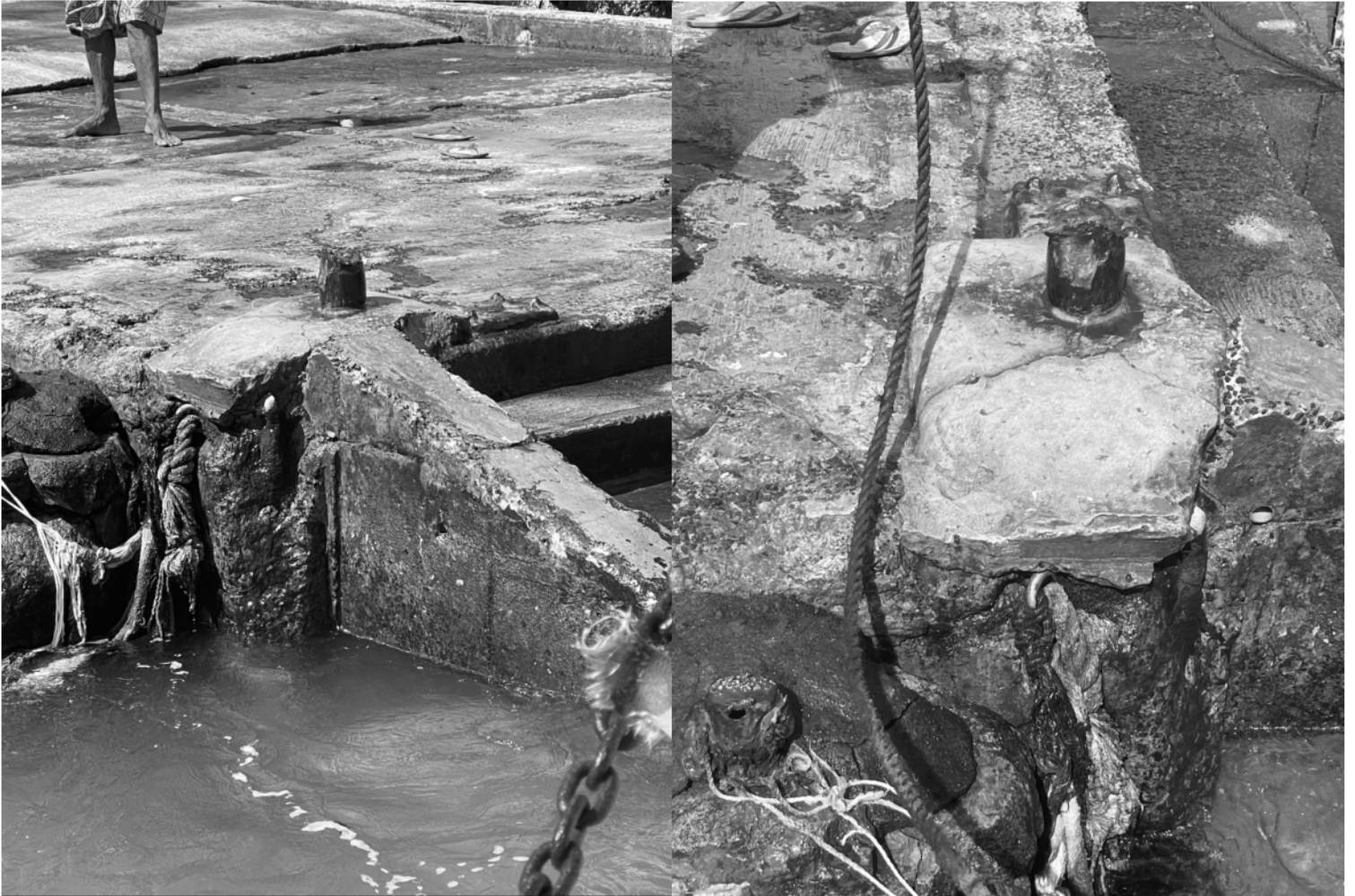
Photo 2 & 3– Shows old cleat that was “ripped” off during operations. It has been left to rust on the wharf and has become a safety hazard. Photos also show strong decay of the wharf structure.
