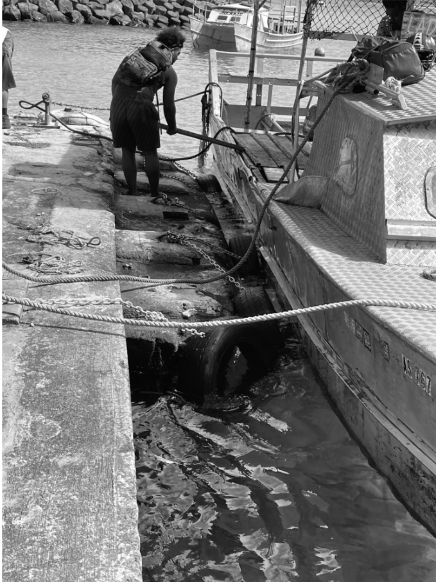
Photo 1 – ASPA Workers getting ready to use wood to unload fuel drums because there is no ramp. Photo shows that the wharf is not in optimum condition for operations. Also shows deteriorating concrete.
