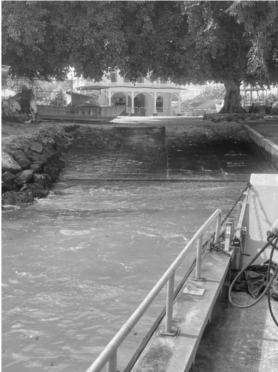
Photo 6 – Shows vast cracking of concrete surface of the ramp. The lack of bollards and cleats on the sides of the ramp make it difficult when tides are strong.
