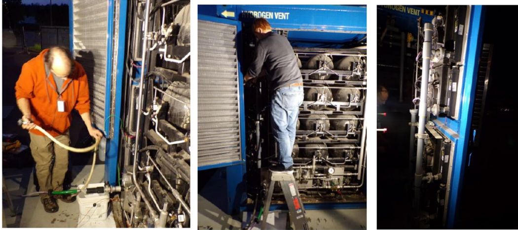
Figure 19. (L) Dave Haywood drains old coolant from the MarFC recirculation system; (M) Max Muller removes broken PVC piping from the MarFC coolant system; (R) the new gray PVC coolant pipe successfully installed.
