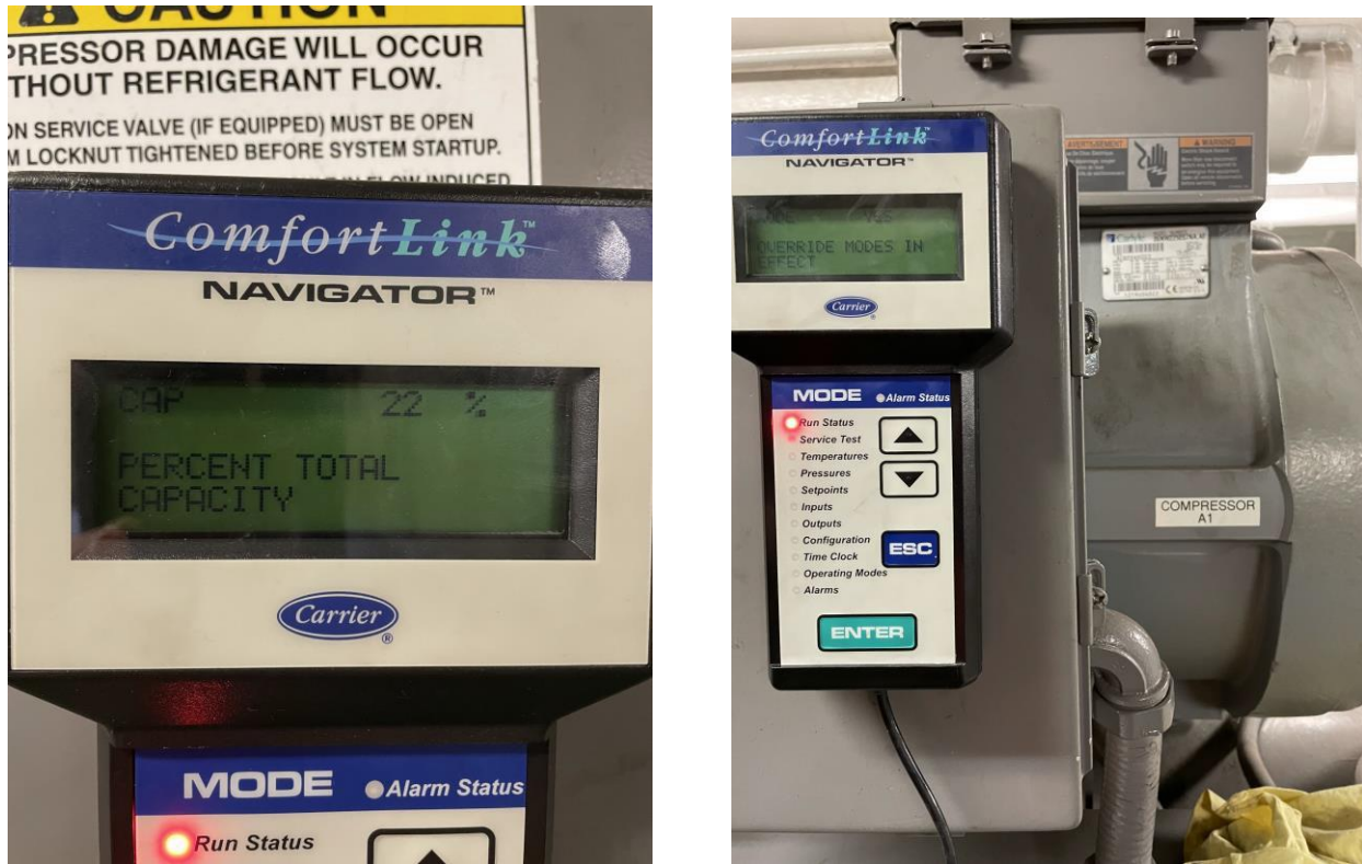
Figure 22 – T/S Golden Bear Onboard Carrier Chiller Display
