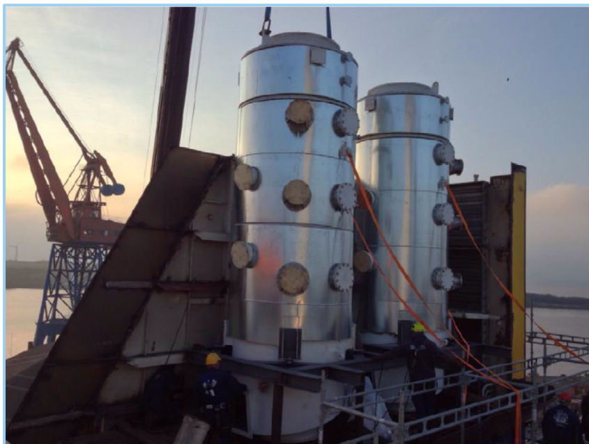
cSO x towers within the funnel space, replacing the silencers
