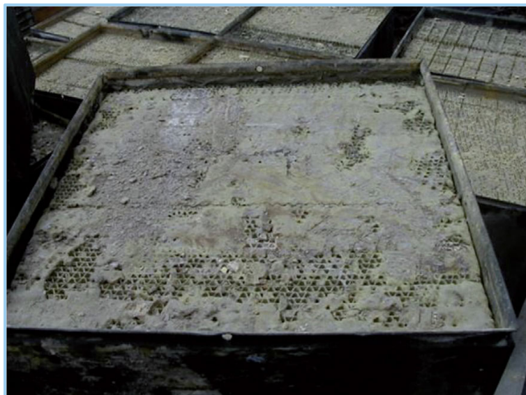
Figure 6 Selective Catalytic Converter, Clogged by Sulfates (Photo by MAN Diesel & Turbo)
