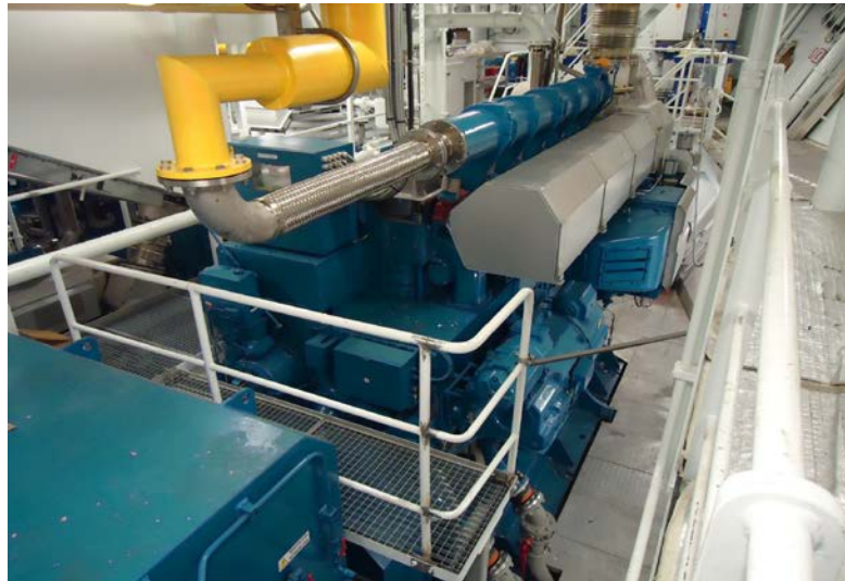
Photo 5: Wärtsilä dual fuel 6L20DF generator set onboard the PSV Viking Princess with double-walled gas supply line in yellow
